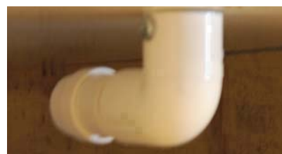
Under the freezer
